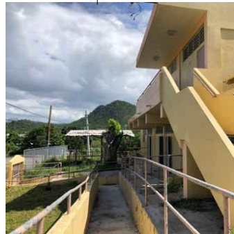
Rampa Too Steep
