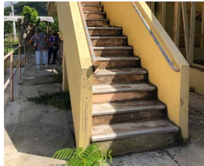
Tight Walkway Adjacent to Stair Between Buildings
